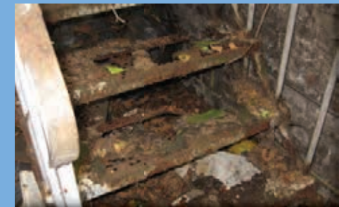
Steel steps after 30 years
